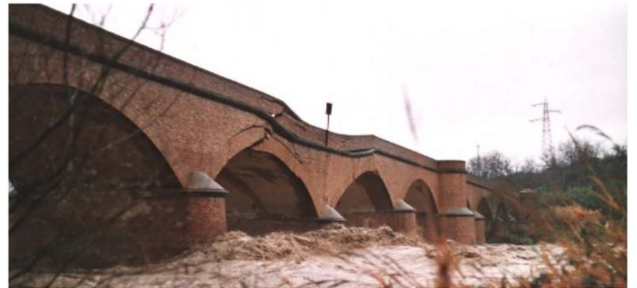
Fig. 1. Collapse of the Trigno river bridge (Italy) during the January 25, 2003 Basso Molise flooding event.
